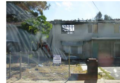
Dwelling damaged by fire in 2008
